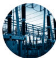
Power Switching Stations
